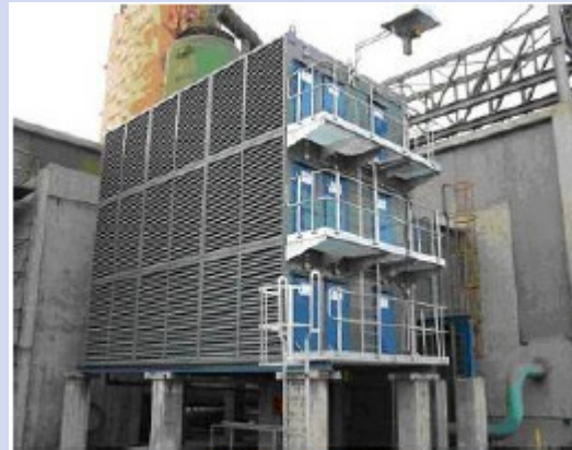
Compressor Air intake
